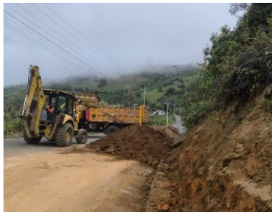
Fig. 4. Landslide at km 14.
