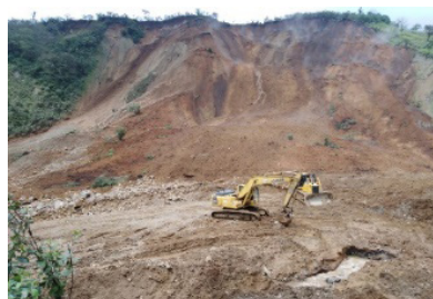
Fig. 3. Landslide at km 13.
