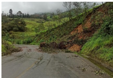
Fig. 2. Landslide at km 3.
