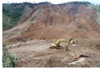
Fig. 3. Landslide at km 13.
