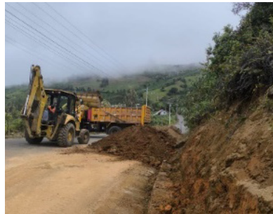
Fig. 4. Landslide at km 14.
