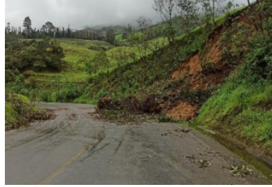
Fig. 2. Landslide at km 3.
